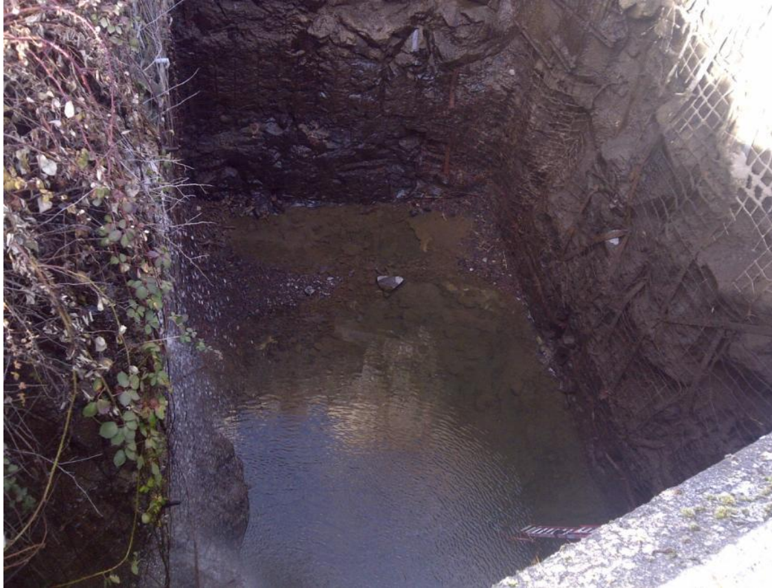
PUD auxiliary water rock plunge pool. To be engineering and geotech inspected Feb 16.
